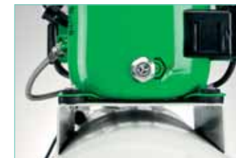
Clearview Oil Level Check
